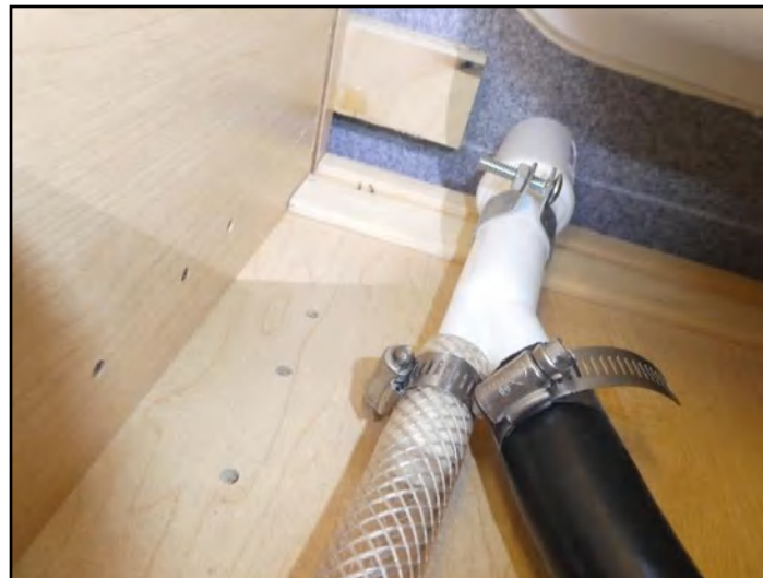
189. Air gap issues
