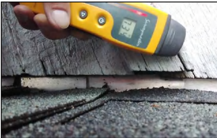
105. High moisture in siding
