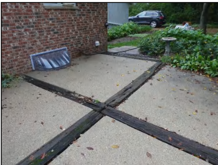
46. Improper slope or drainage
