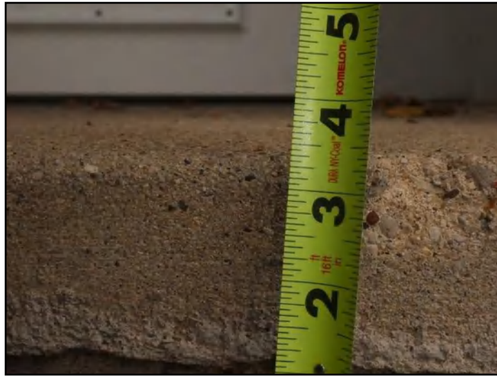
45. Improper slope or drainage
