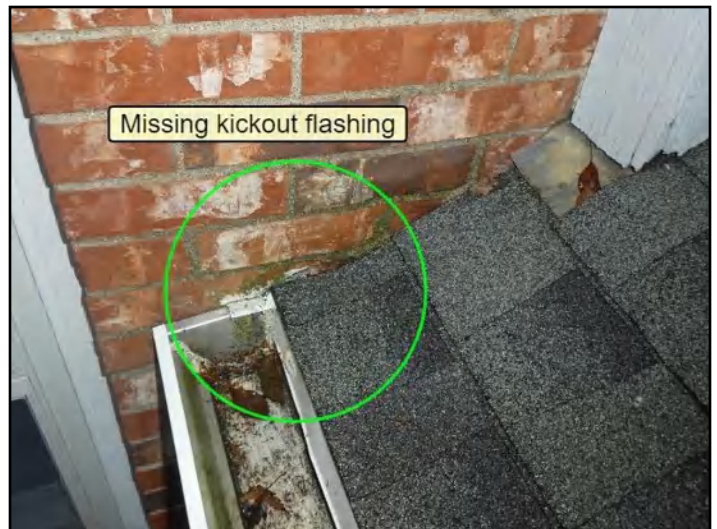
91. No kick-out flashing
