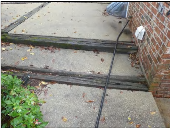
48. Improper slope or drainage
