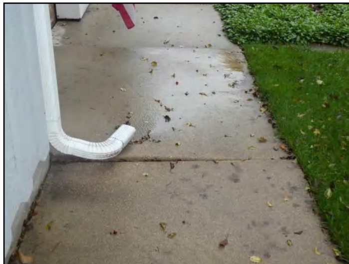
96. Downspout discharges on sidewalk. This...
