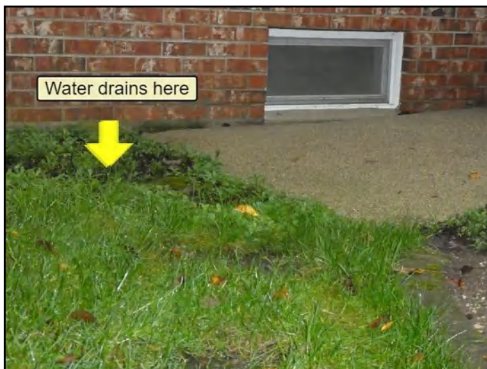
50. Improper slope or drainage
