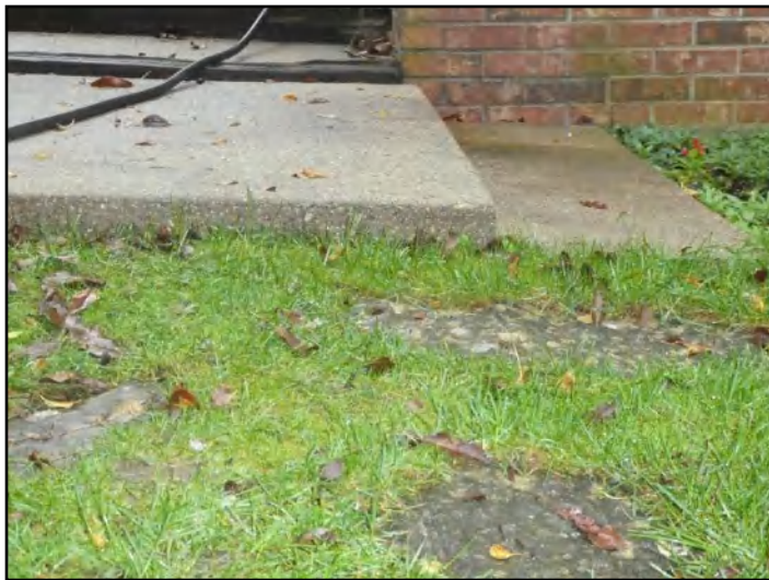
49. Improper slope or drainage
