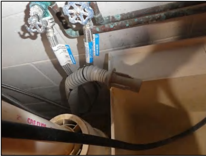
82. Missing stand pipe
