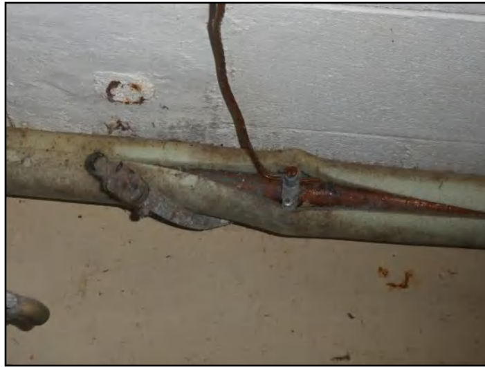
146. Copper - water pipe
