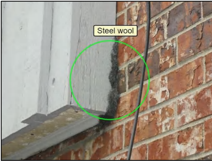
14. Steel wool being used to prevent animal entry
