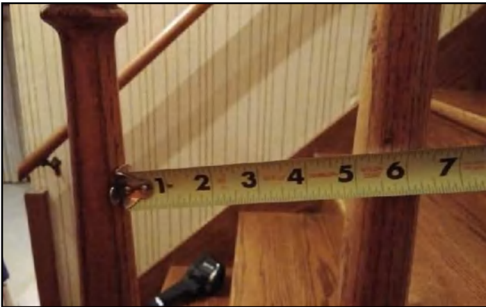
113. Spindles (balusters) too far apart
