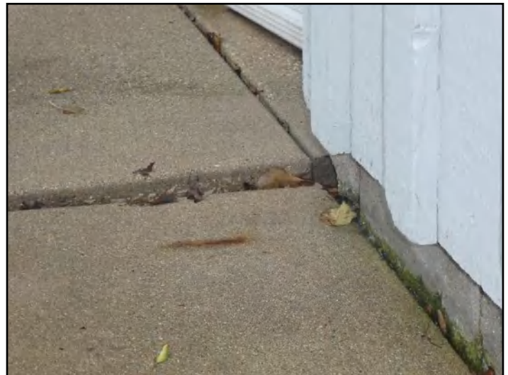
125. Improper slope or drainage
