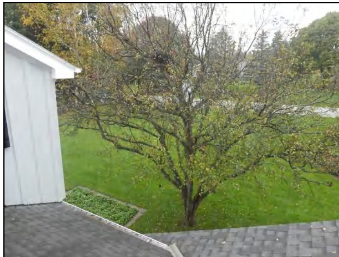
121. Trees to close to house. Trim back.
