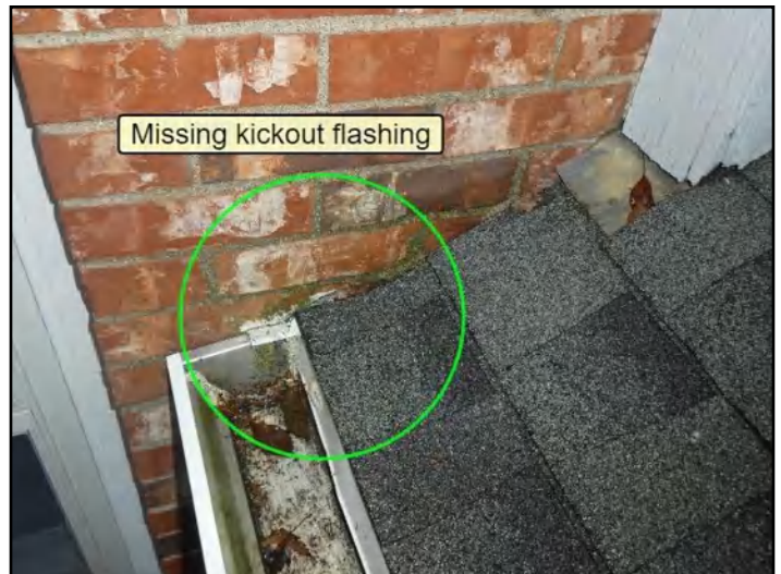
8. No kick-out flashing
