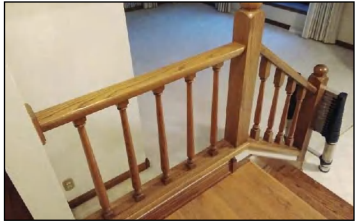
33. Spindles (balusters) too far apart
