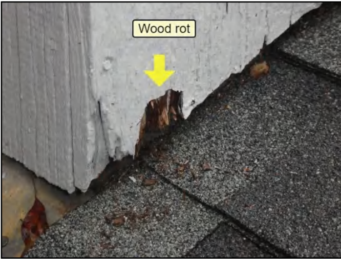
107. High moisture in siding
