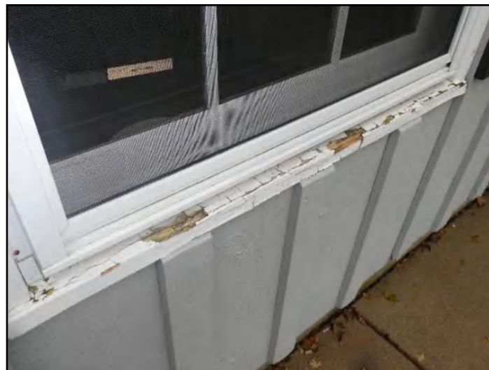
29. Rotting window sill
