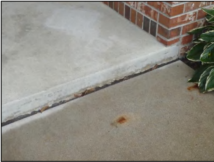
126. Improper slope or drainage
