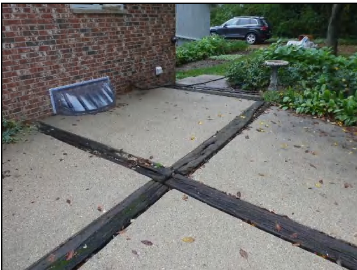
131. Improper slope or drainage
