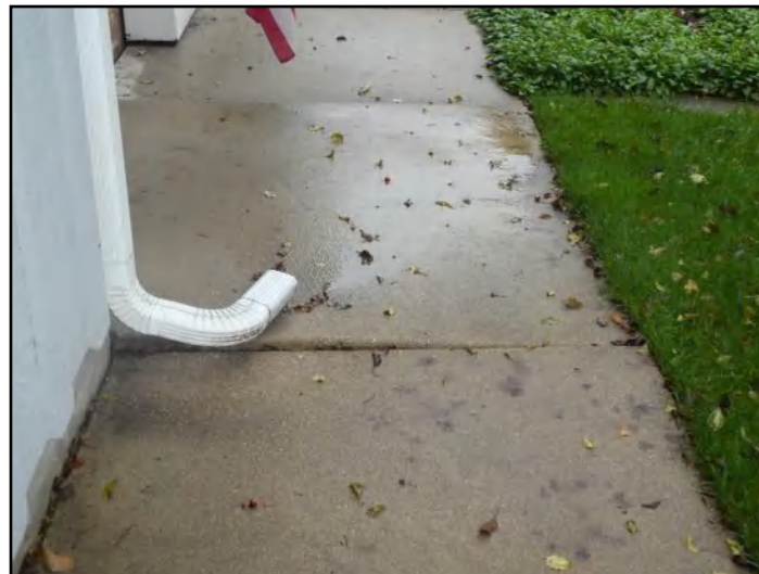
13. Downspout discharges on sidewalk. This...
