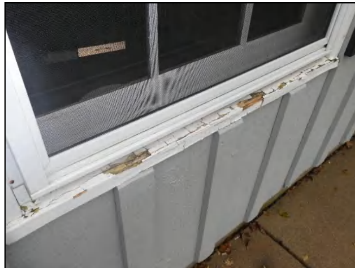
112. Rotting window sill
