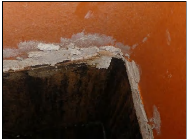
61. Poor flue repair
