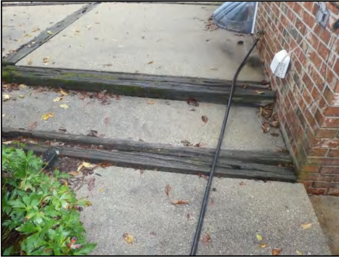
133. Improper slope or drainage
