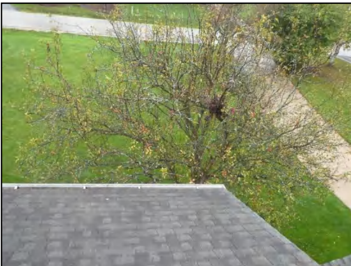
117. Trees to close to house. Trim back.
