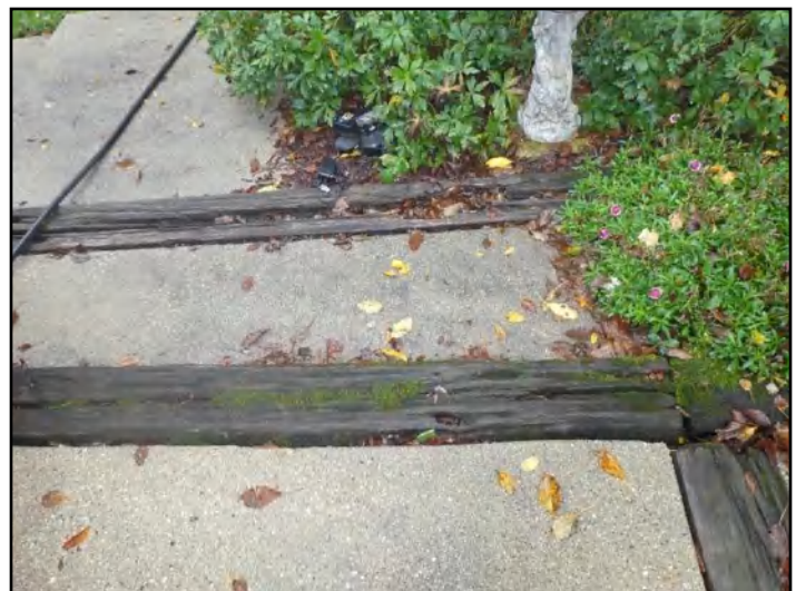
47. Improper slope or drainage
