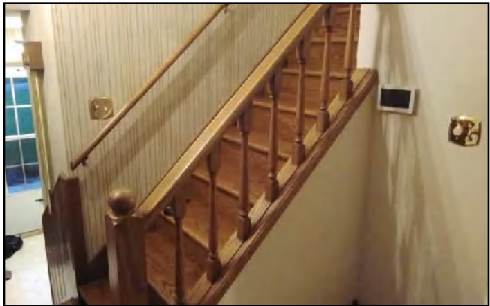
31. Spindles (balusters) too far apart
