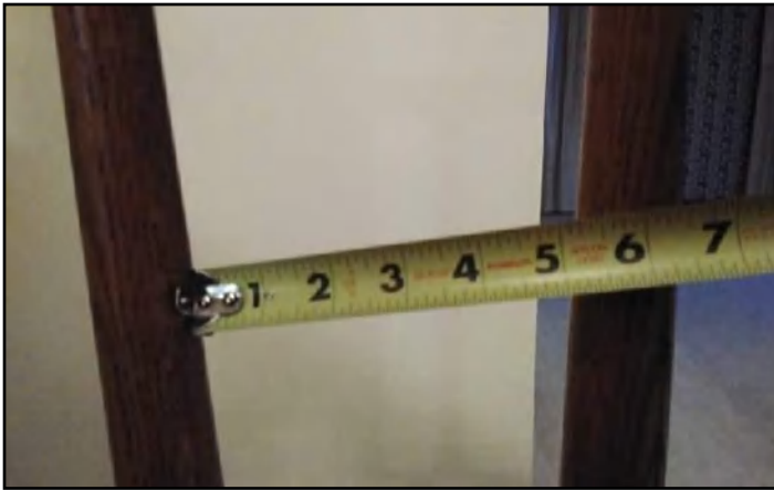
32. Spindles (balusters) too far apart
