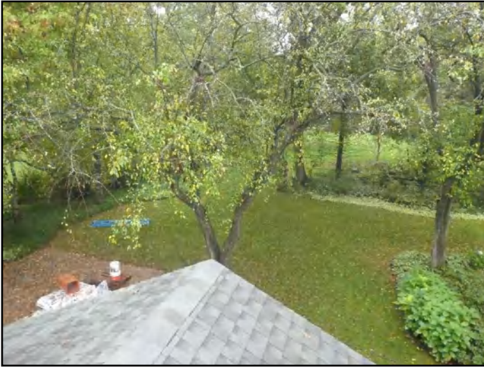
36. Trees to close to house. Trim back.
