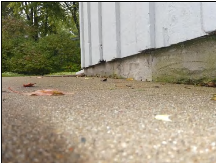
124. Improper slope or drainage
