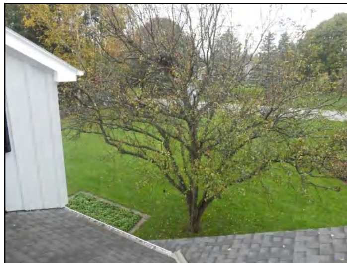
38. Trees to close to house. Trim back.
