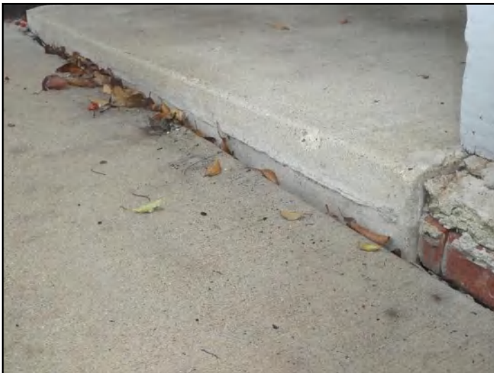
43. Improper slope or drainage
