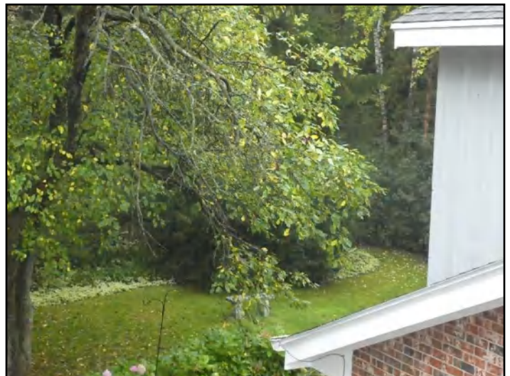
35. Trees to close to house. Trim back.
