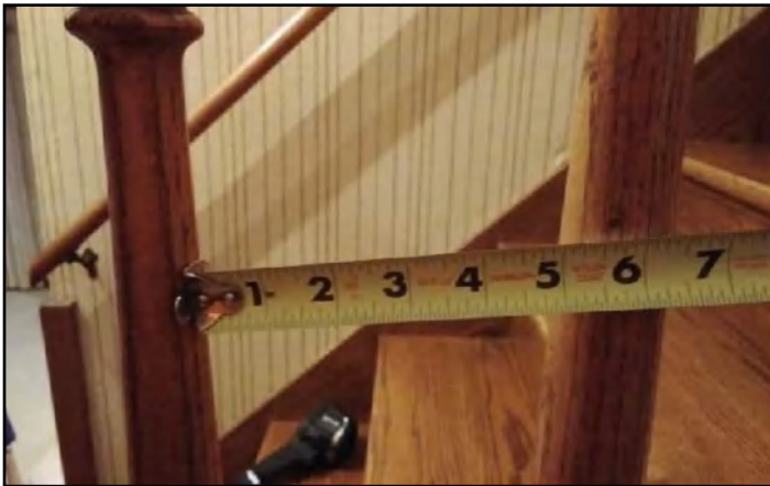
30. Spindles (balusters) too far apart
