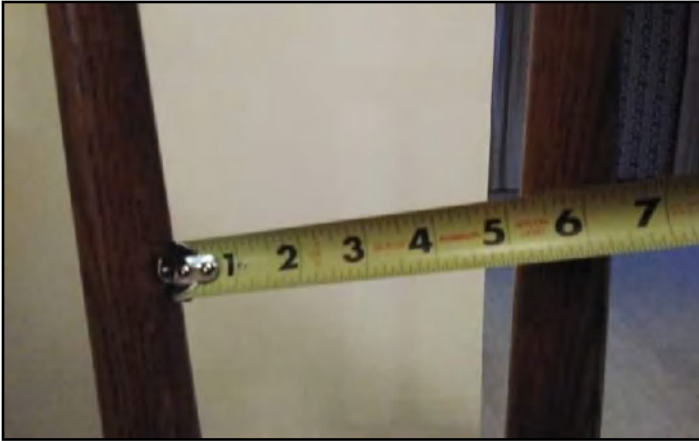
115. Spindles (balusters) too far apart
