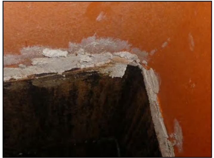
150. Poor flue repair
