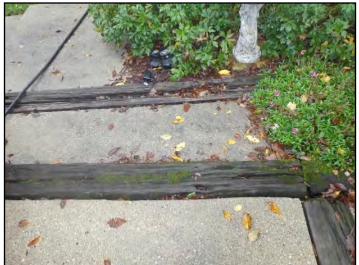
132. Improper slope or drainage
