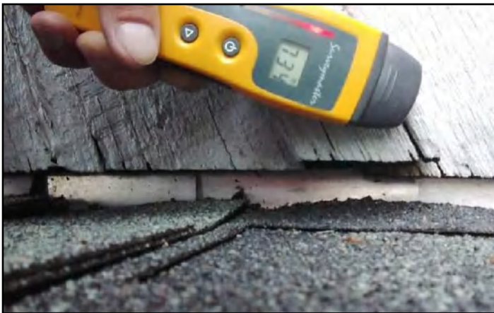
22. High moisture in siding
