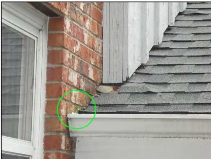
7. No kick-out flashing
