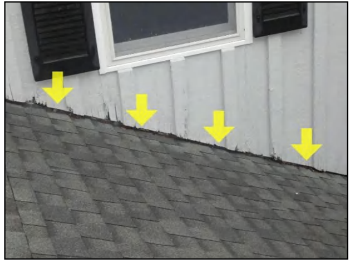
25. High moisture in siding
