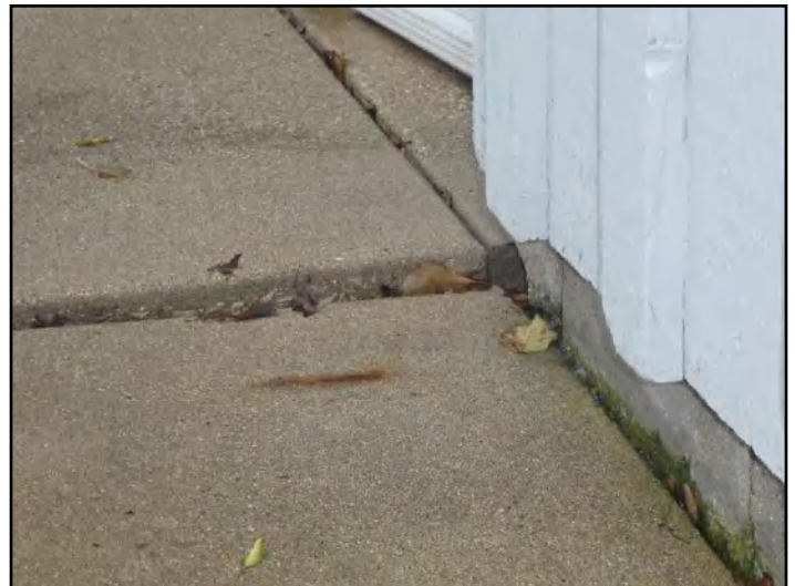
40. Improper slope or drainage
