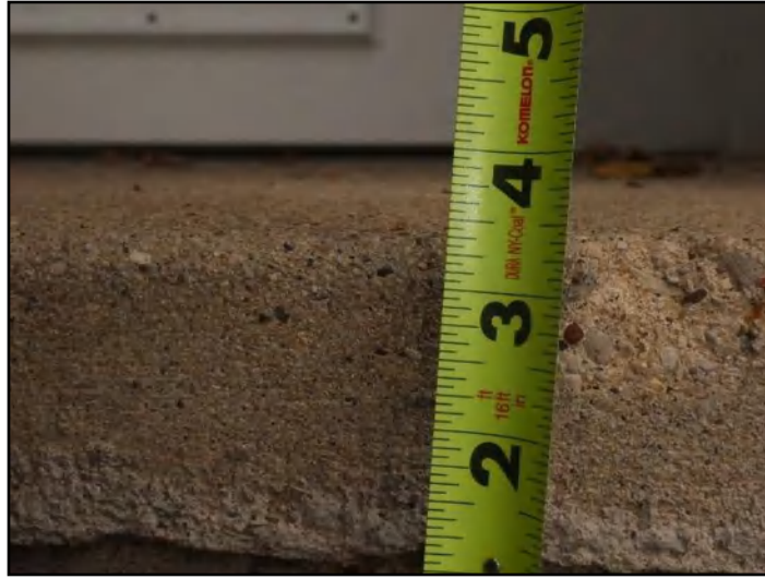
130. Improper slope or drainage
