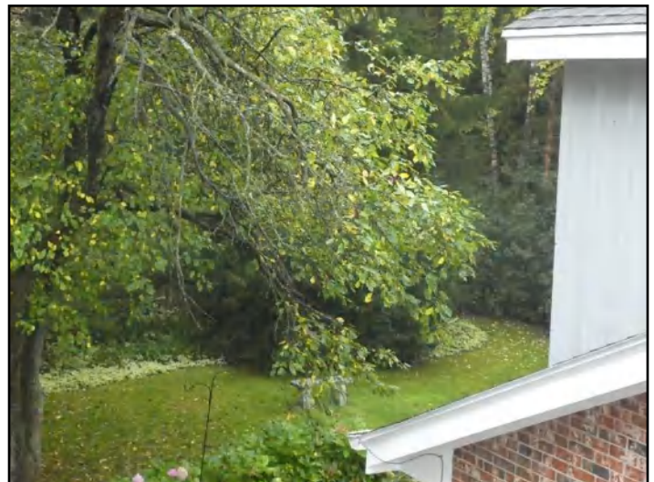
118. Trees to close to house. Trim back.
