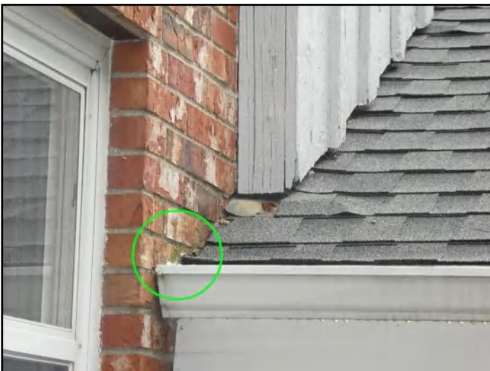
90. No kick-out flashing
