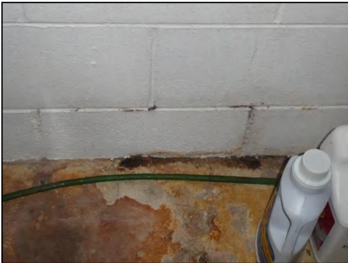
137. moisture on foundation wall
