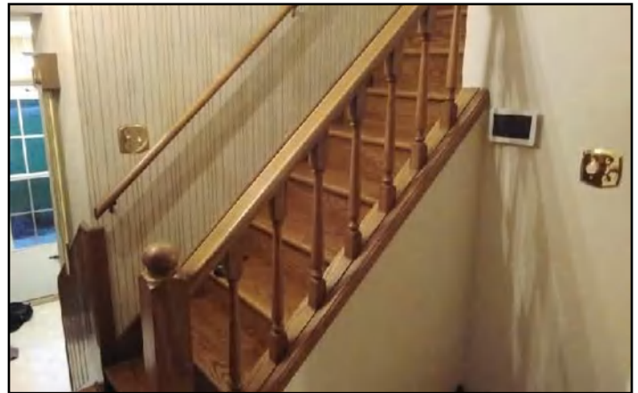
114. Spindles (balusters) too far apart
