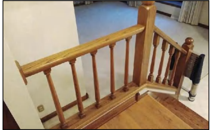
108. Spindles (balusters) too far apart
