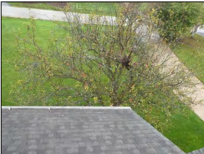
34. Trees to close to house. Trim back.
