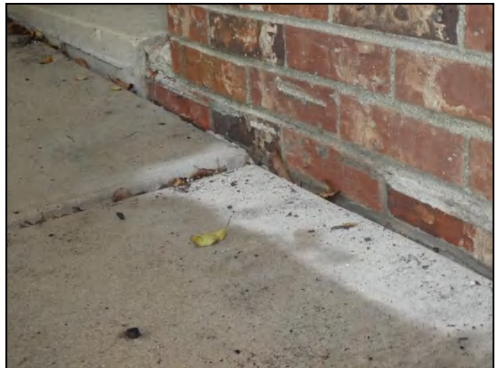
44. Improper slope or drainage
