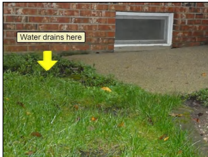
135. Improper slope or drainage
