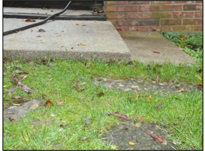
134. Improper slope or drainage
