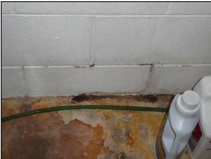
51. moisture on foundation wall
