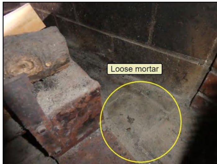
154. Deteriorated, missing or loose masonry or...
