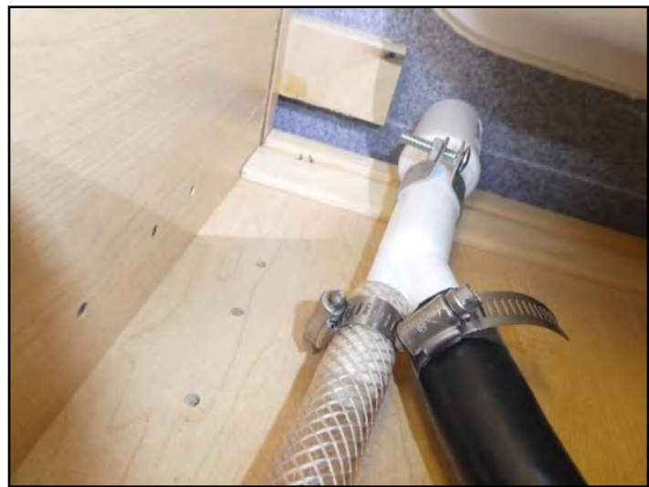
81. Air gap issues
