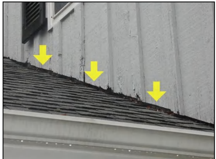
106. High moisture in siding
