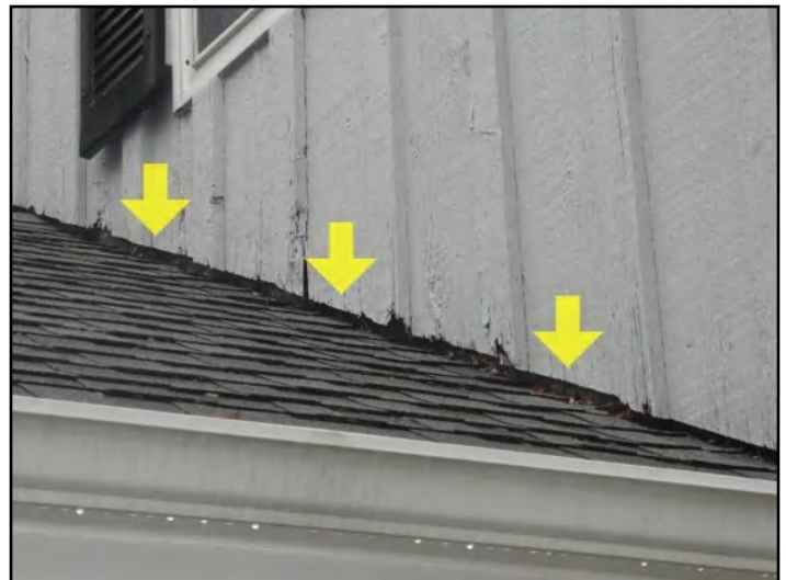
23. High moisture in siding
